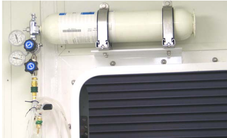
Figure 2-13. Calibration Sample Gas Cylinder
