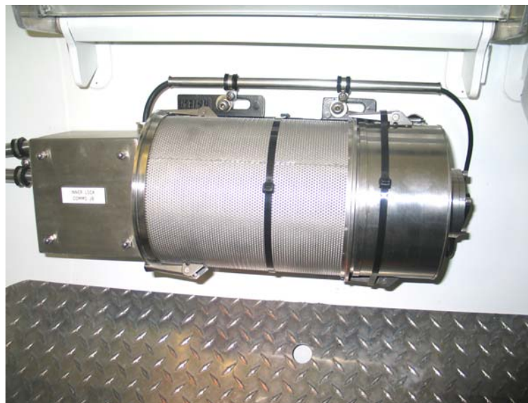
Figure 3-21. Carbon Dioxide (CO 2 ) Scrubber Assembly
