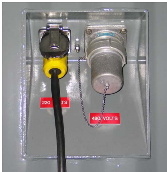
Figure 2-2. Power Receptacle Box
