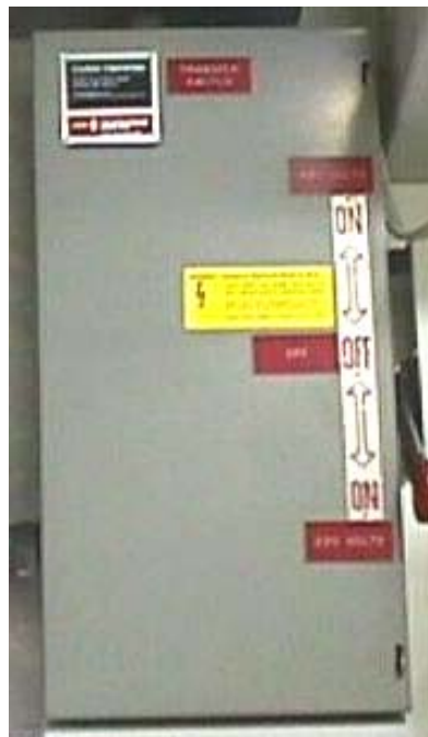
Figure 3-2. Manual Bus Transfer (MBT) Switch
