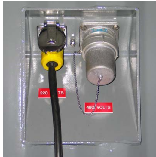
Figure 3-1. Power Receptacle Box
