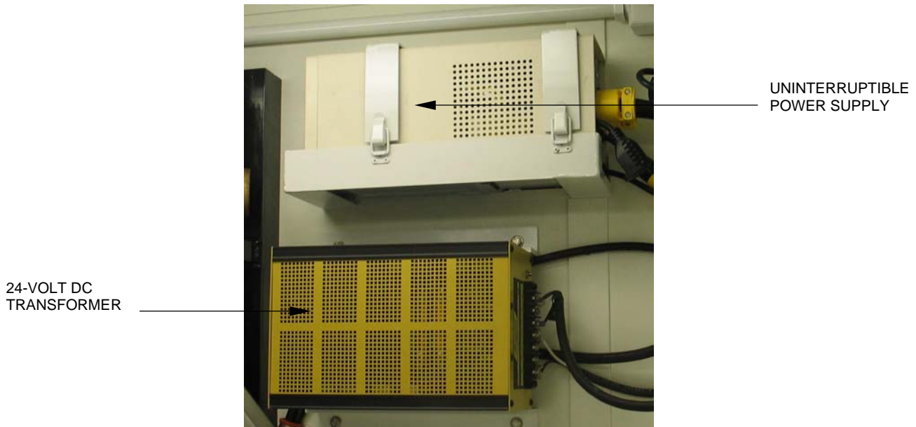
Figure 3-4. Uninterruptible Power Supply and Transformer
